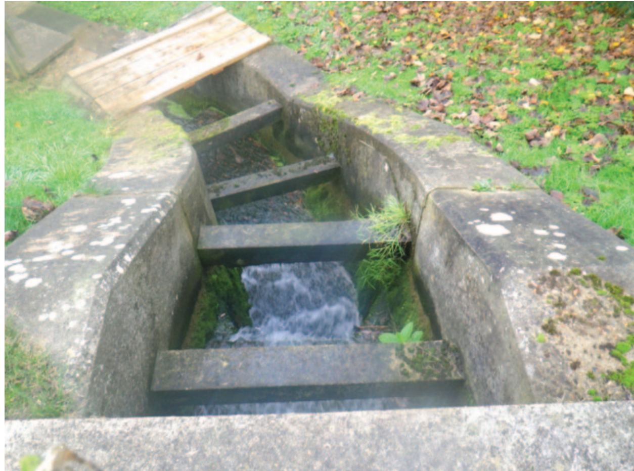
The water falls by approximately 6 metres via a weir as it exits the millpond
